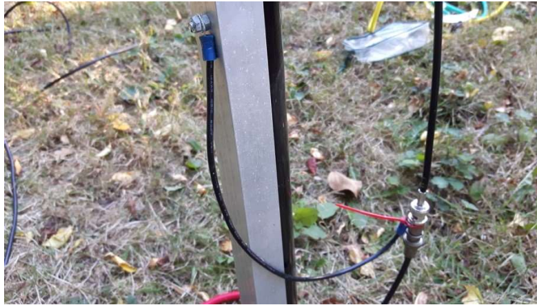
Fig 5 – Grounding of Coax Braid at base of support
